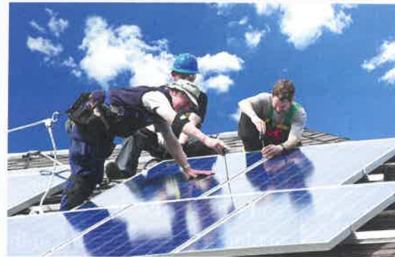
▲ Solar power installation
